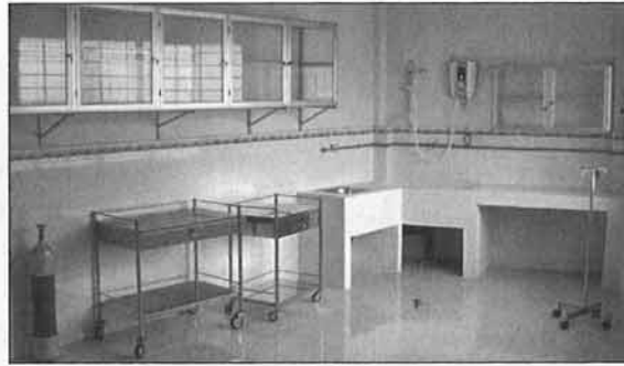
THE ENTIRE GO VAP ORPHANAGE was recently remodeled including the bathrooms, left, and the emergency room, right.
